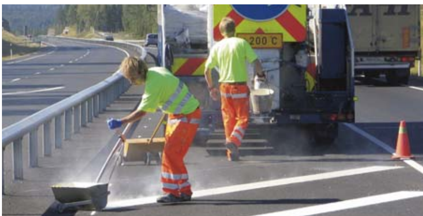
For the Highway 9 paving contract Lemminkäinen supplied mineral aggregates, asphalted the road and carried out the road-marking works. At over one hundred kilometres in length, the highway section between Orivesi and Jyväskylä is the longest unbroken stretch of road ever paved under a single contract in Finland.
