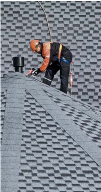
Reducing the number of workplace accidents is one of the most important aims of Lemminkäinen's safety work.
