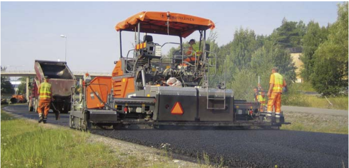
Particular attention was paid to life cycle costs, pavement performance characteristics and environmental effects in the design and construction work on Highway 9 near Turku.
