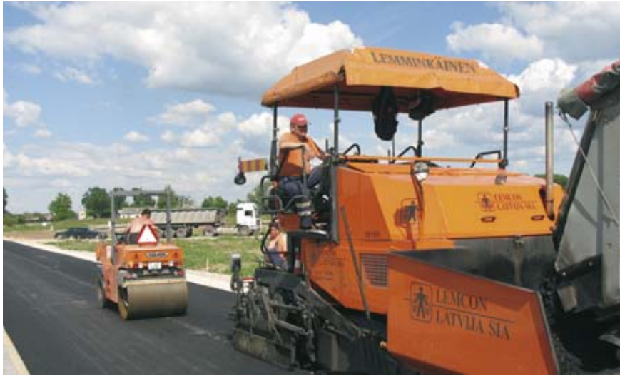
Asphalt paving work on the streets in a new residential area of Sigulda in Latvia.
