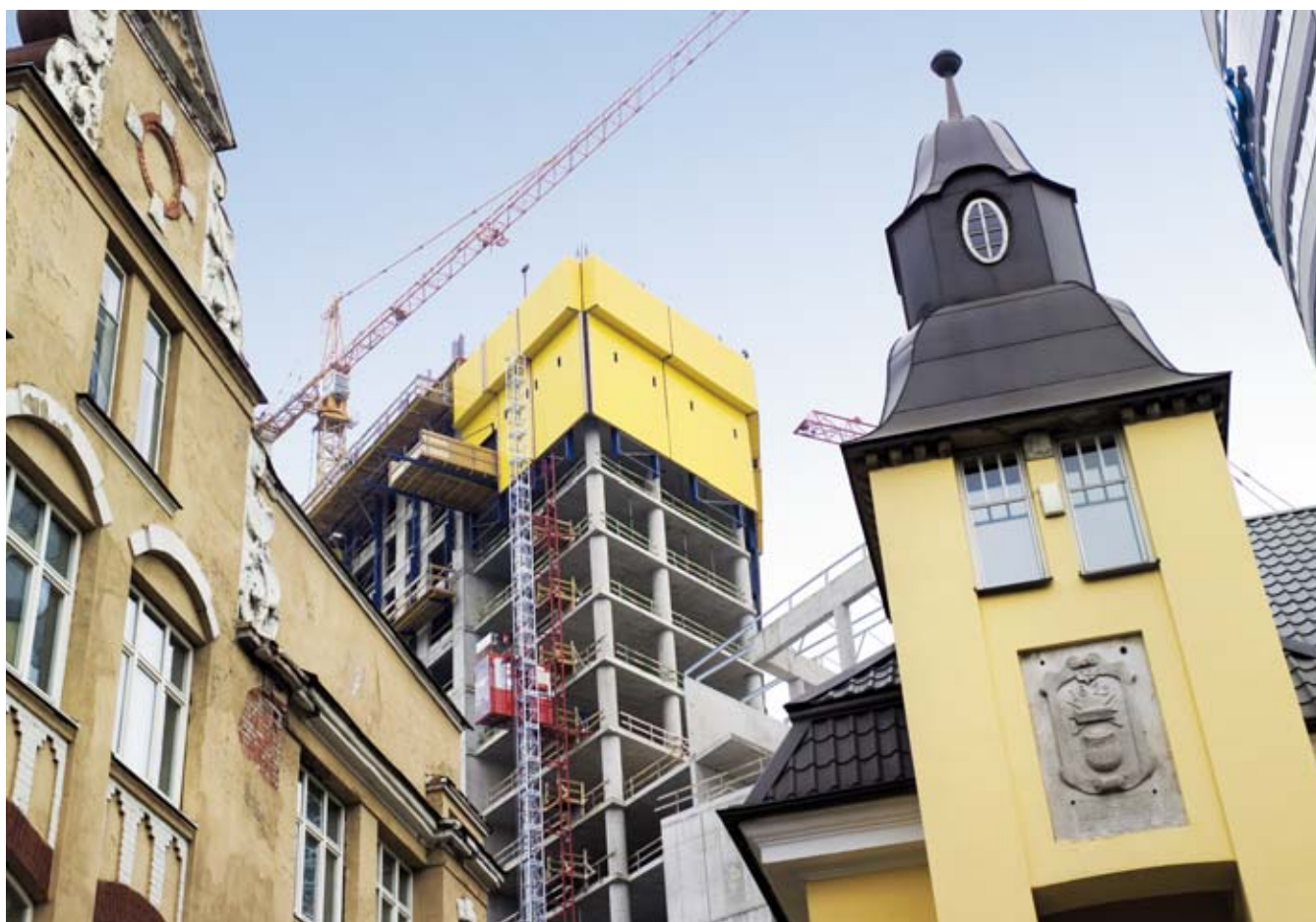
The installation of protective wall elements keeps pace with the rise of the skyscraper in Tallinn. The panels prevent objects from falling and provide shielding against the wind.
