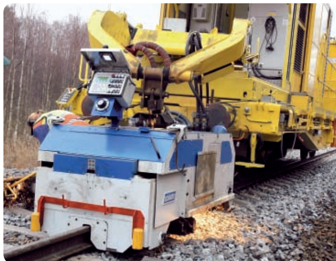
VR-Track commissioned a new type of flash butt welding machine that joins rail ends by heating them with electric current. This new welding method is fast and the welded joint is more durable.
