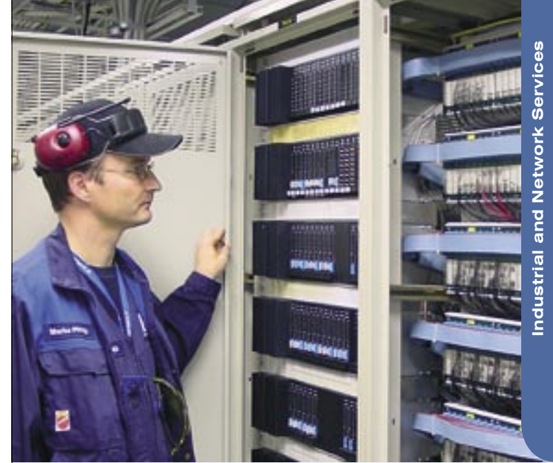
Automation installer Marko Pihlaja inspecting the measurement data of a soda recover boiler at Metsä-Botnia's pulp mill.
