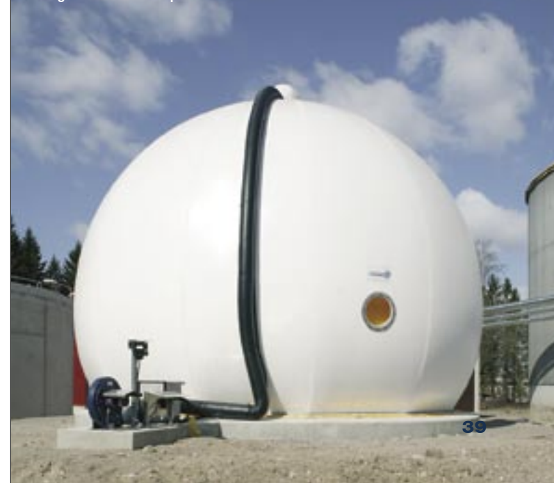
The extension of the Riihimäki wastewater treatment plant upgrades the efficiency of water treatment in the city of Riihimäki and at the Valio dairy. The methane gas generated by the anaerobic digestion process is stored in a gas bell and utilized for electricity and heat generation at the plant.
