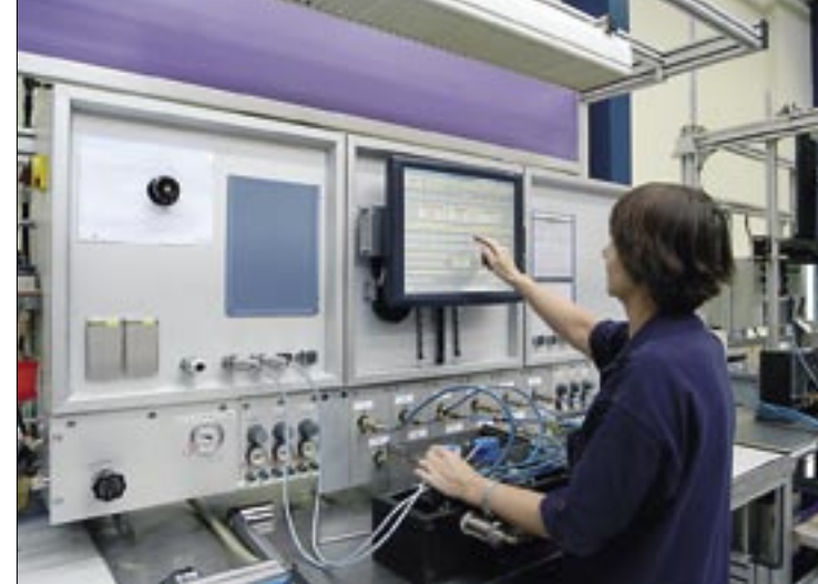
Control equipment and data collection systems supplied by YIT are used to test valves at the Danfoss valve plant in Kolding, Denmark.
