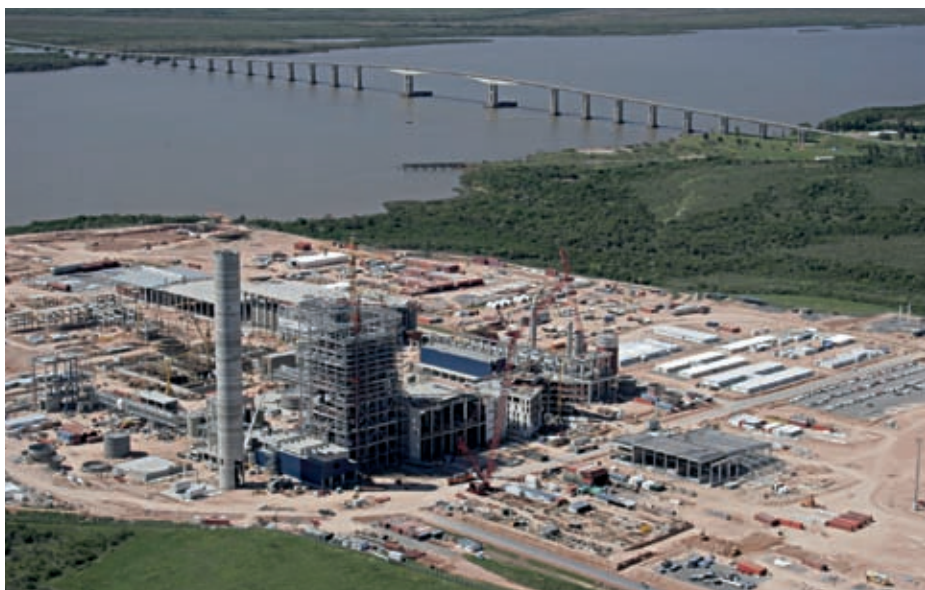
Lemcon is building a pulp mill for Botnia at Fray Bentos in Uruguay.
