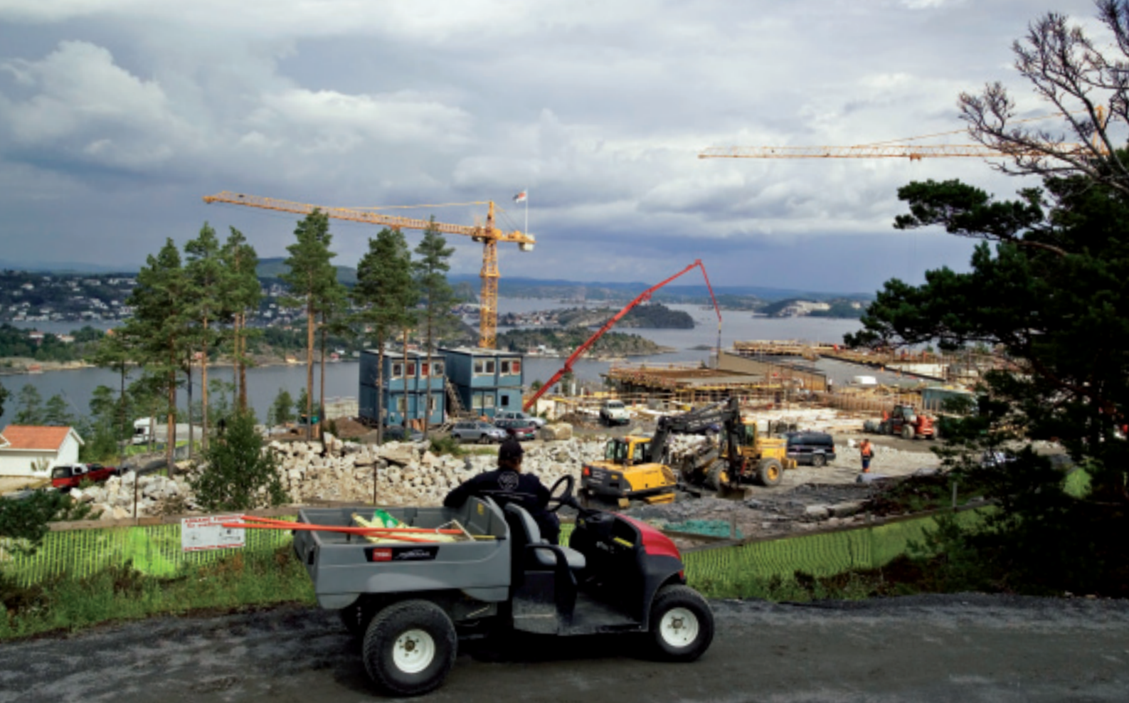
Onninen delivers materials to SPA and Golf hotel construction site in Kragerø, Norway.
