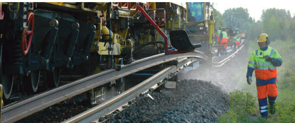
VR-Track's biggest superstructure project of the year was on the Turku to Toijala line.
