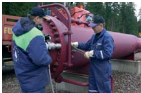
Gasum is responsible for network maintenance.
