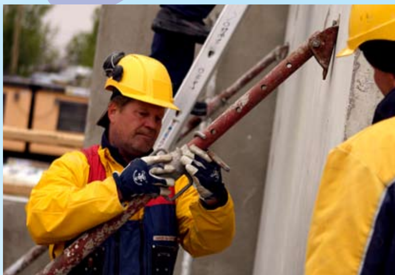
Jorma Vehviläinen at work as a supervisor of a group installing prefabricated concrete slabs at the construction company Palmberg.
